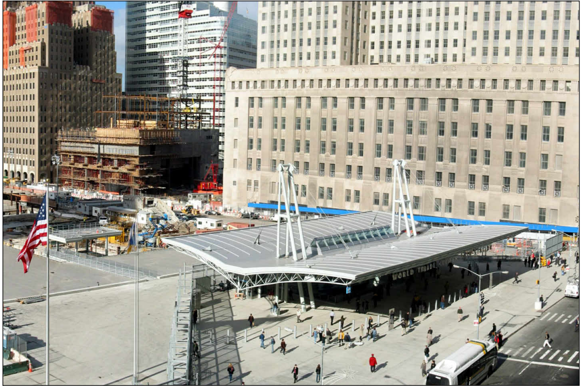
View northwest of the WTC Site showing the temporary WTC PATH station. 7 WTC is under construction in the background
