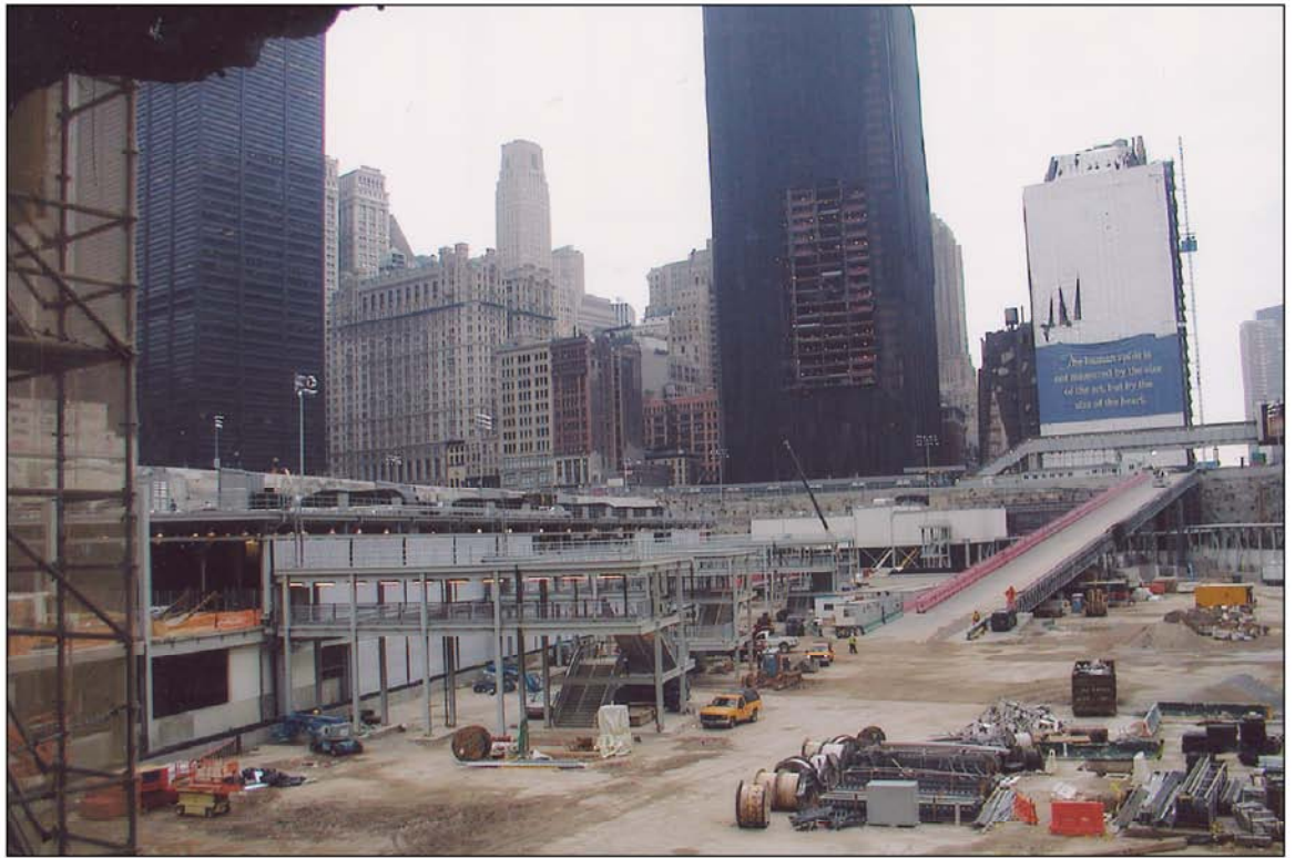
View southeast of the WTC Site, showing the temporary WTC PATH station on the site 1
