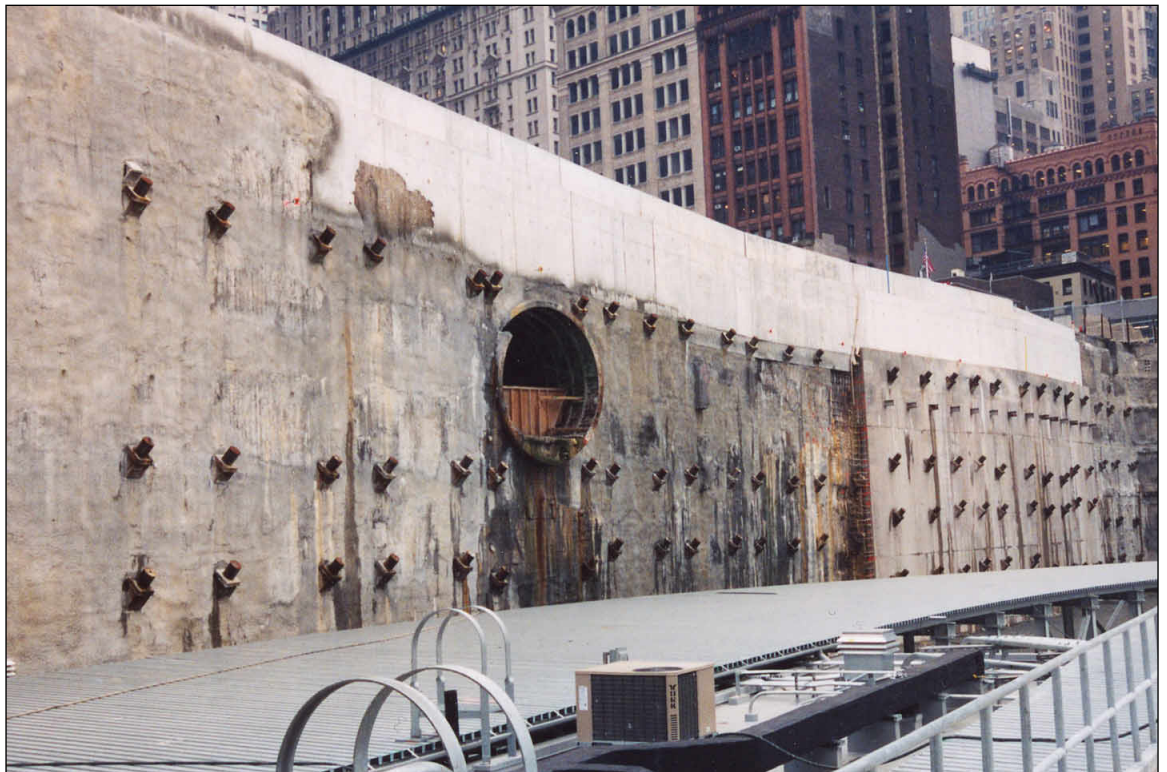
View showing remaining portions of the Hudson Tubes in the eastern slurry wall
